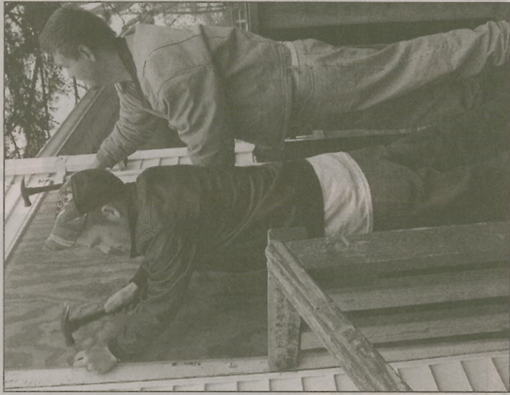
Josh Keen and John Cope board up a side door at a vacant house on Atlantic Street NE.
